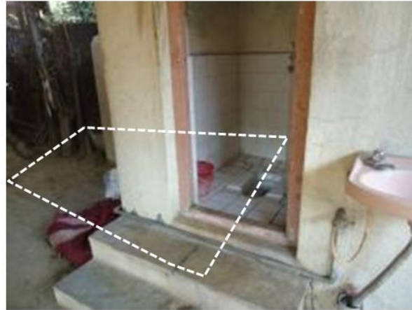
Inaccessible septic tanks with sealed tops
