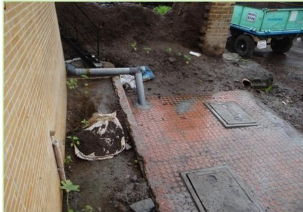
Oversized septic tanks
