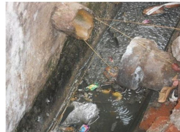
Toilets directly connected to drains
