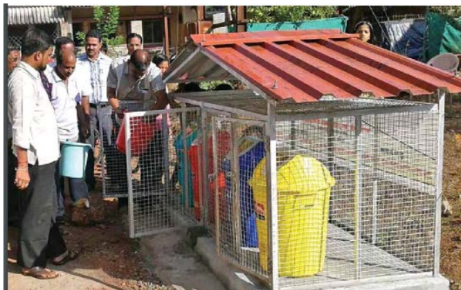
Photograph 8 Dustbins for disposal of segregated waste
