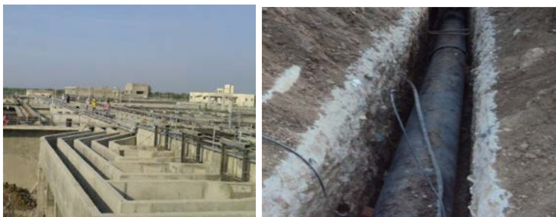
L: STP in construction in Jamnagar, R: laying of UGD lines in Vadodara
