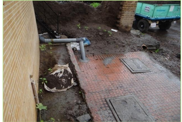
2 Chambered septic tanks located behind community toilets
