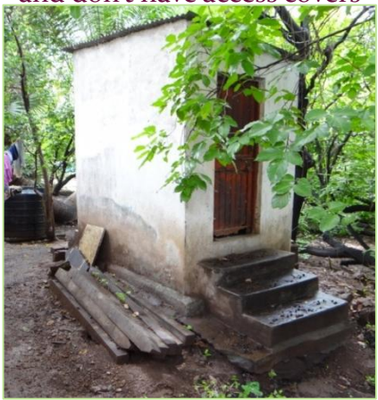
Septic tanks are below the toilets and don't have access covers
