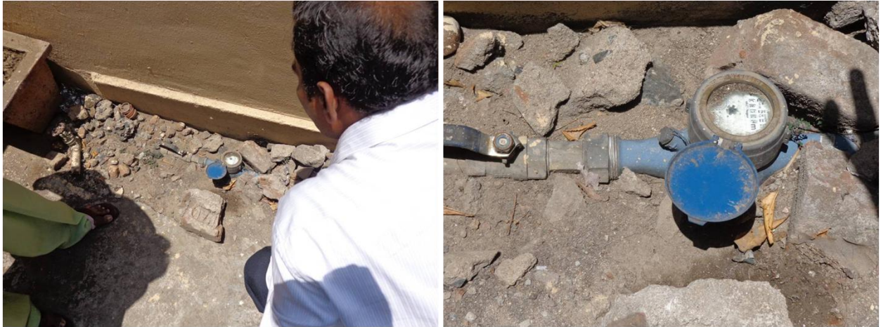
Consumer meters installed in the front yards of buildings
