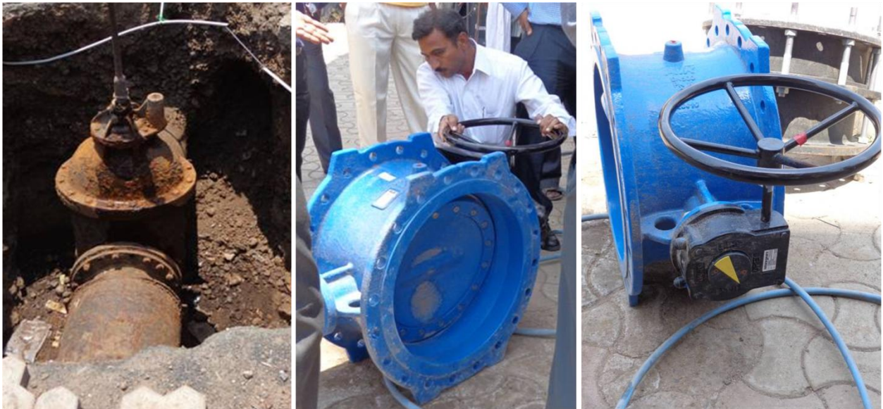
Replacement of Valves at WDS with Potential to operate the new Valves using actuators via internet or SMS
