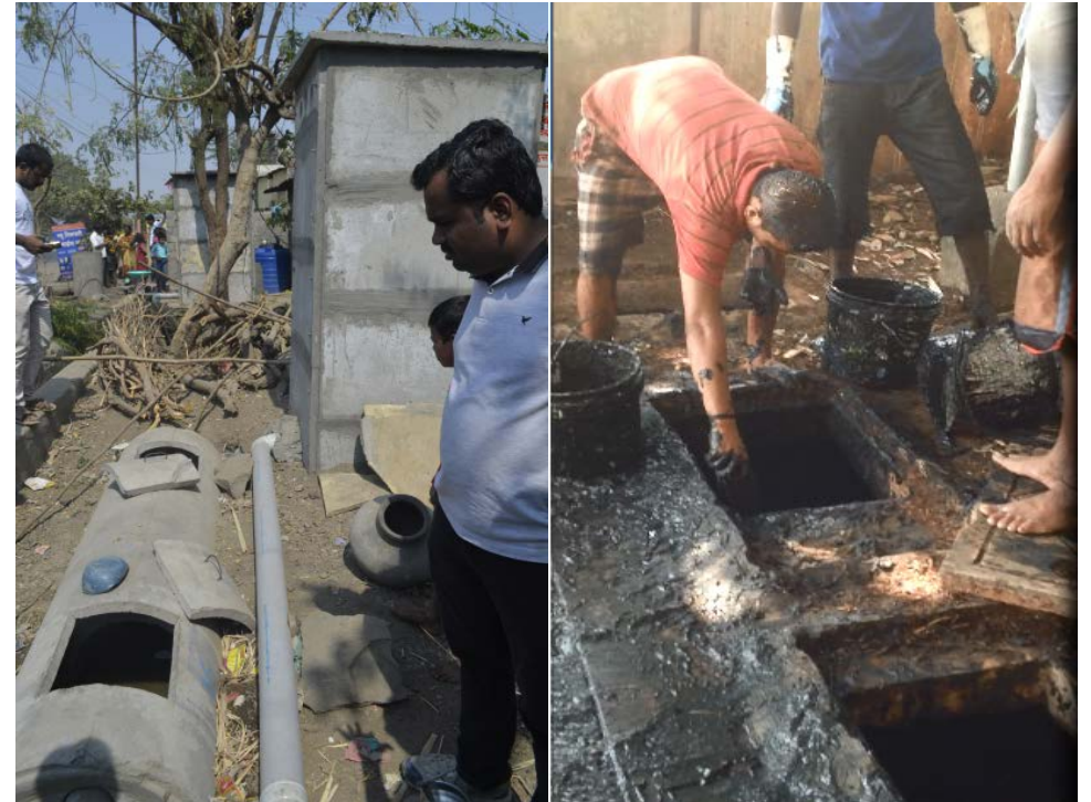
Newly installed septic tanks in Sangola MC (on left) and Septic tank emptying by people in Alibaug MC (on right)
