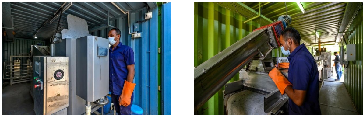
Figure 5 Operations at Wai FSTP
