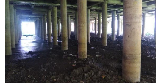
Figure: Location Below STP where sludge from centrifuge is disposed
