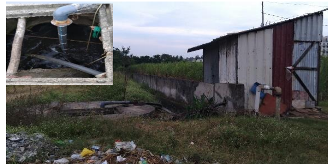
Figure: Pumping Station install by farmers to reuse treated wastewater from Kasaba Bawada STP through the chambers at treated wastewater drainage pipeline
