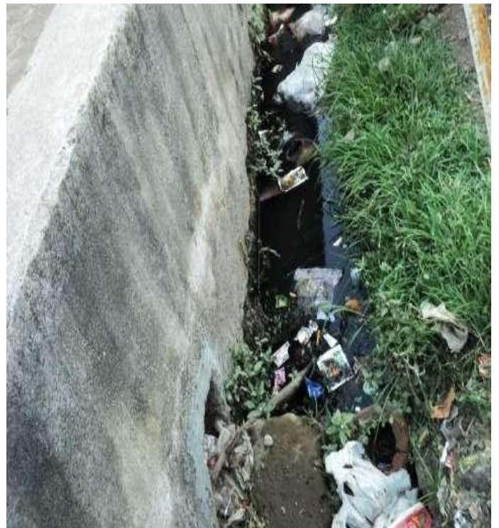
Widespread clogging of drains
