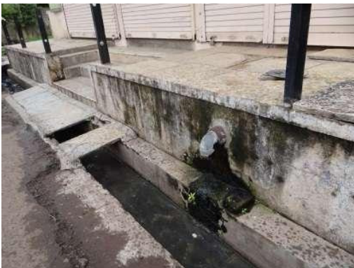
Effluent and grey-water being discharged into drains
