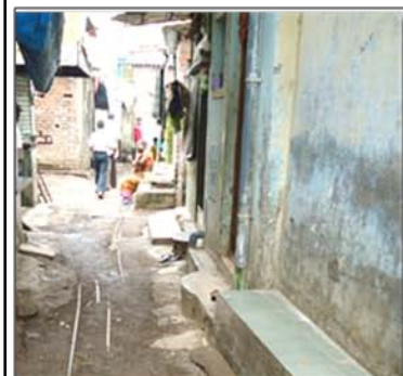
Internal water supply network in slum I
