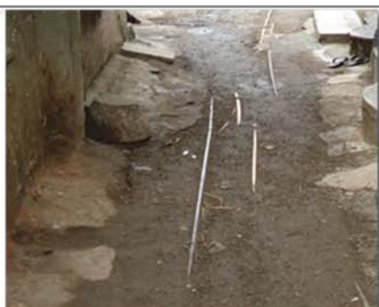
Internal water supply network in slum I I
