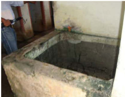
Water Storage outside Community Toilet
