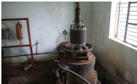
Pumping station at AMC
