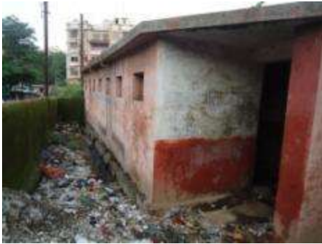
Non functional community toilet
