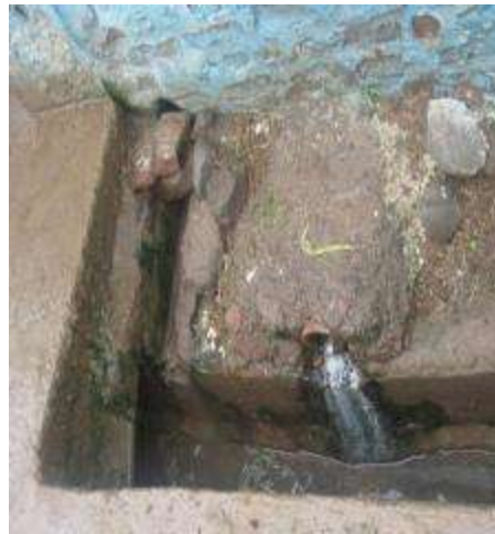
Sullage disposed in open drains
