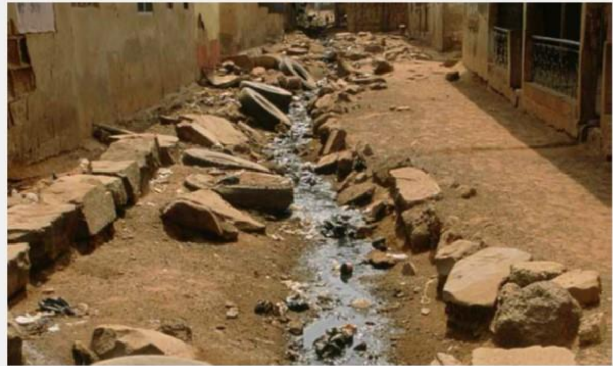
An open sewer in between houses, Woriziehi, Tamale, Ghana.
