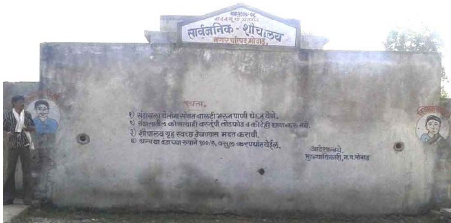
Photograph 4: Instructions for users on CT wall of ward no 7
