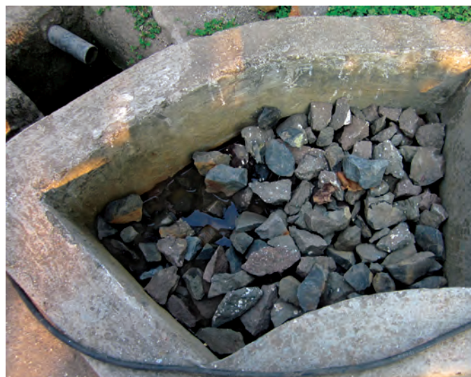
Inlet zone with filter media
