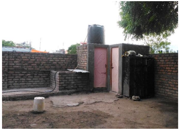
Vandana has completed construction of toilet and bathroom. An overhead water tank is placed since the area does not have piped water supply. Cost of construction of the toilet was approx. Rs 50,000. She has borrowed Rs 15,000 from ICICI bank.
