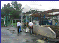
Mechanised Dewatering Unit : 8 Nos
