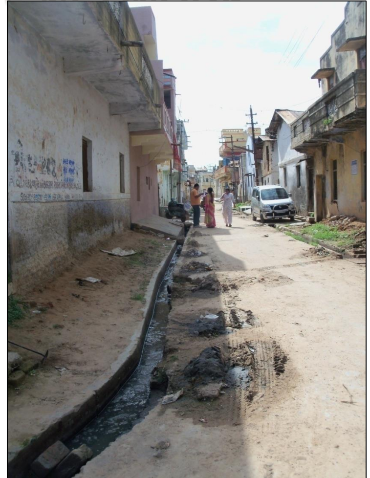
Open drain in Mansa
