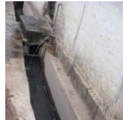
Clean drains in Wai Municipality that carry storm water and grey water
