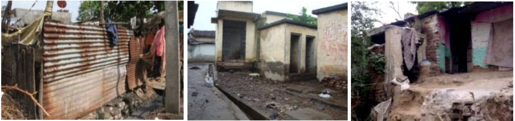
Condition of individual toilets in slums, Maharashtra
