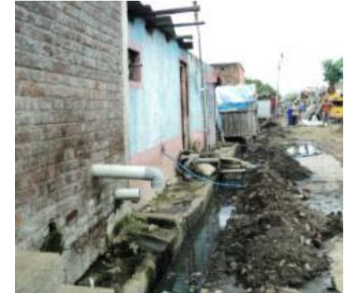
Septic tank effluents flowing in open drains in Hingoli Municipality
