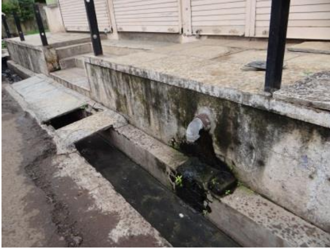
Effluent and grey-water being discharged into drains
