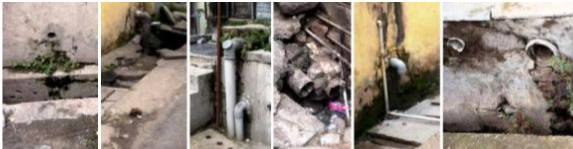
Blackwater/effluent from septic tanks is discharged into natural drains.
