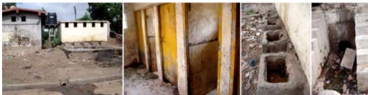
The condition of some community toilets in Indiranagar slum in Sinnar.
