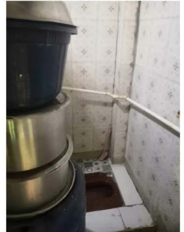
Household toilet connected to unscientific septic tank
