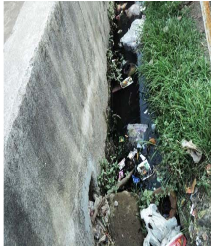
Widespread clogging of drains
