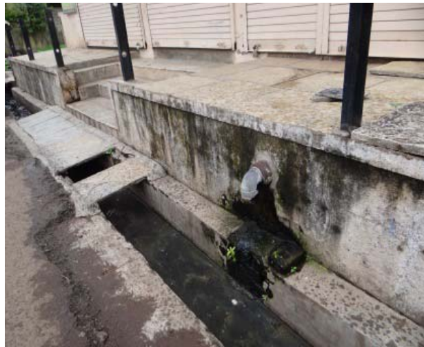
Effluent and grey-water being discharged into drains
