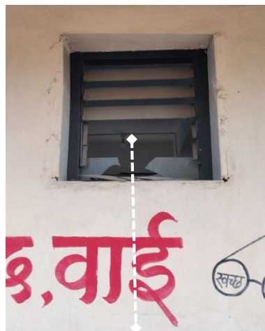
Broken Windows in female cubicles
