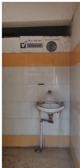
A wash basin is provided at the entrance, but there is no soap facility provided.
