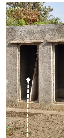
Broken Doors in newly built female cubicles
