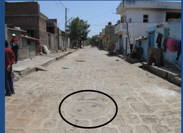
Sewer line installed in slum but not operational
