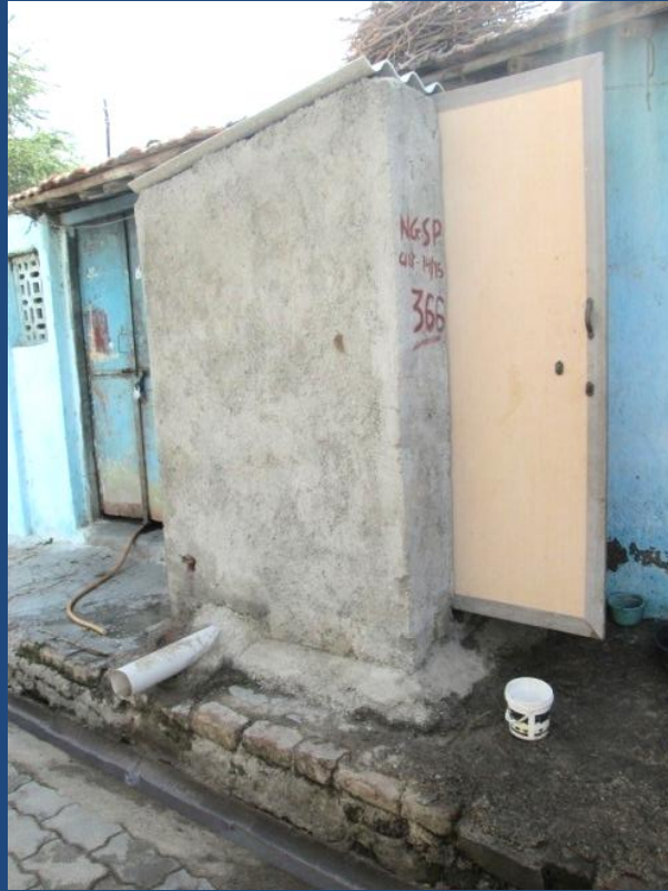
Toilet not connected with disposal system
