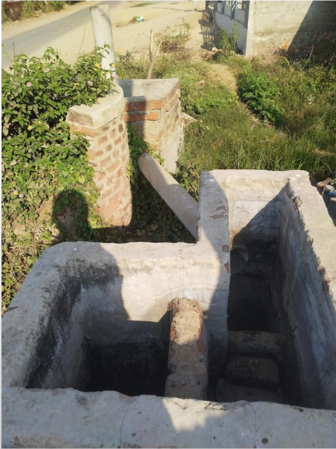
Desludging chambers are misaligned.
