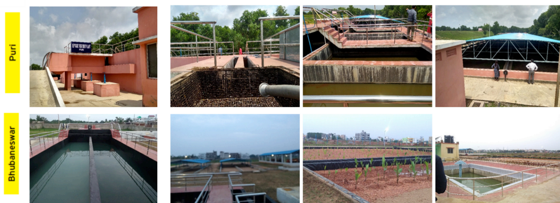
Figure 42 Treatment Plants in Bhubaneswar and Puri, Orissa
