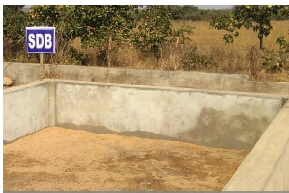
Figure 3: Levelled sand surface of SDB Source: Ner, Amravati FSTP
