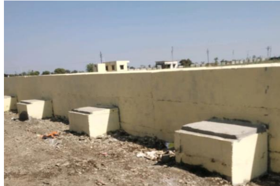
Figure 8 Maintaining effluent collection chambers Source: Risod FSTP (C-WAS)
