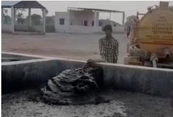
Figure 5: Facilitating flow of sludge on to splash pad Source: C-WAS
