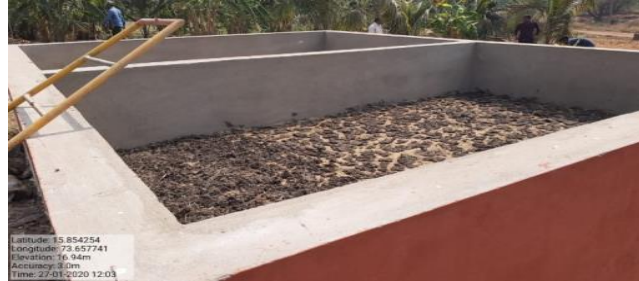
Vengurla Sludge drying bed
