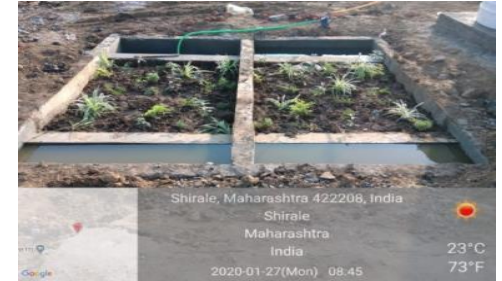
Peth Planted gravel filter
