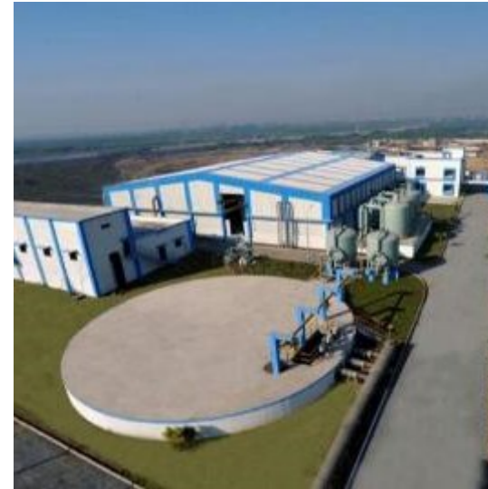
Tertiary Wastewater treatment plant
