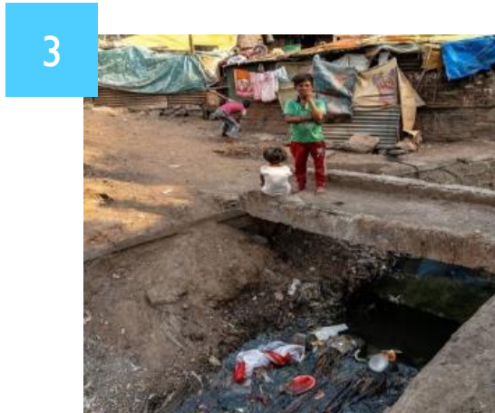
Upgradation of open surface drains to closed drains for storm water drainage
