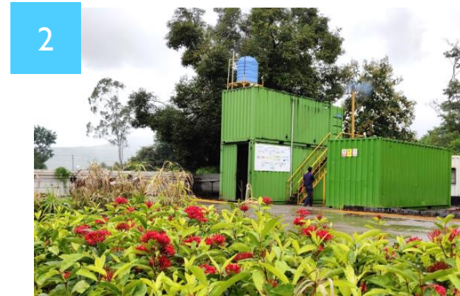
Operation and Maintenance of Fecal Sludge Treatment Plant
