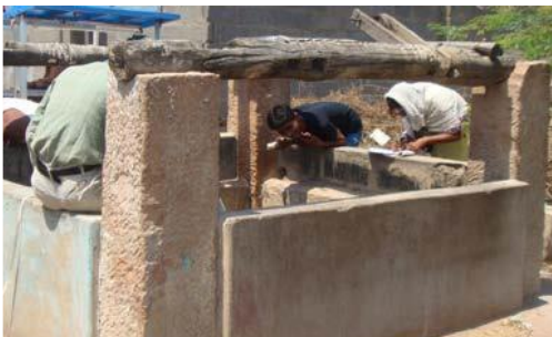
Revival of old unused well for decentralized piped supply for a slum
