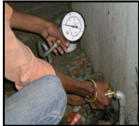
24x7 meter and valve fixing
