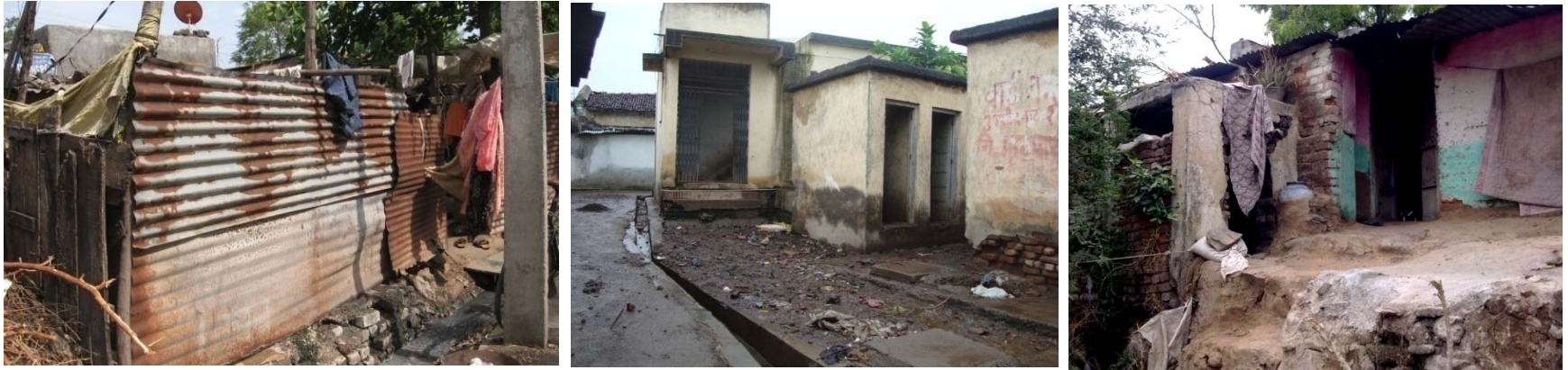
Condition of individual toilets in slums, Maharashtra
