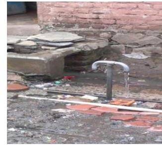
Public Standpost in Yavatmal
