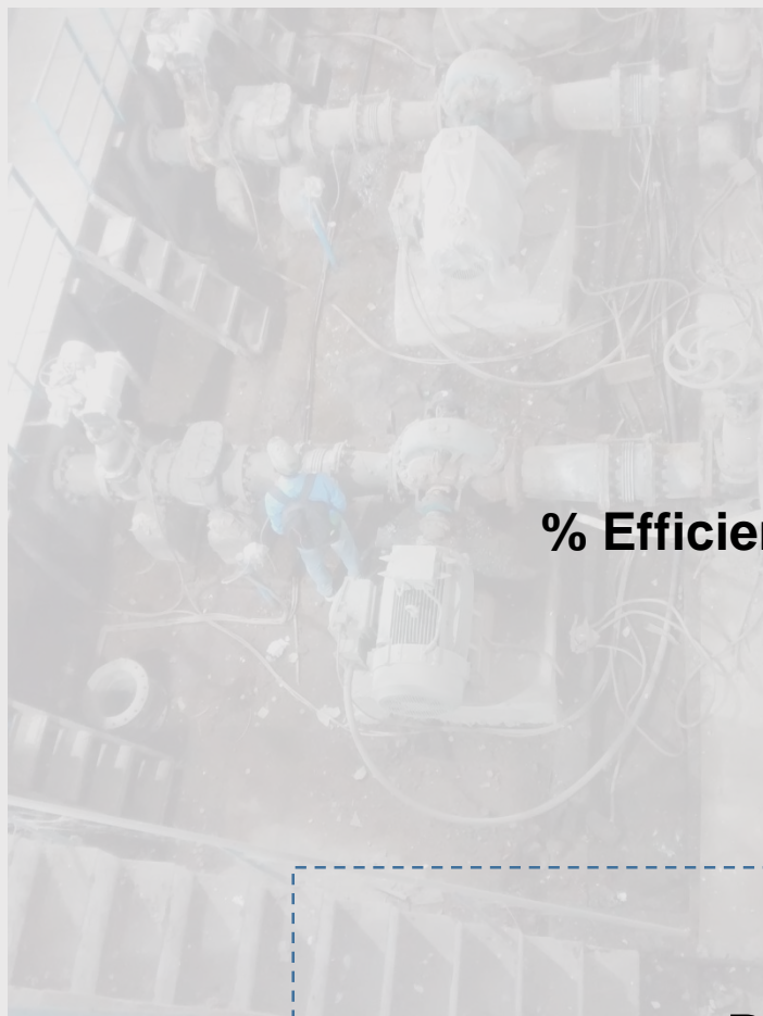
Lal Darwaza Water distribution station
