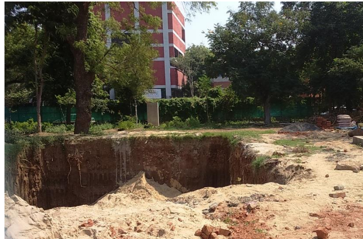
Storage Tank For Treated Water
