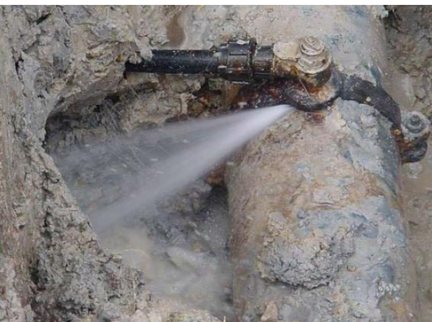
Thousands of small leaks go undetected
