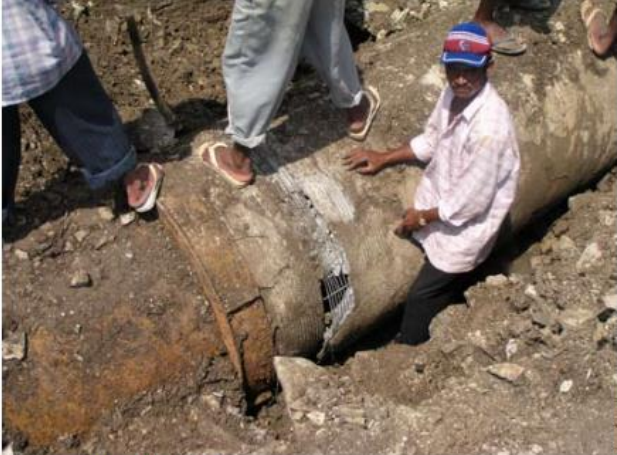
Poor infrastructure condition is a major problem
