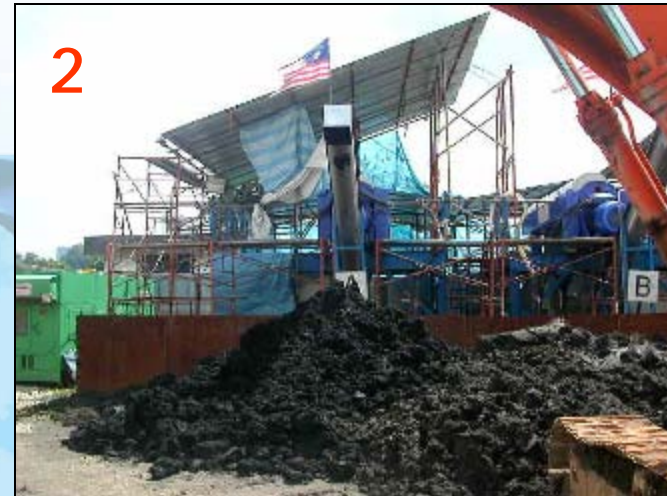
Dried Sludge after Dewatering
