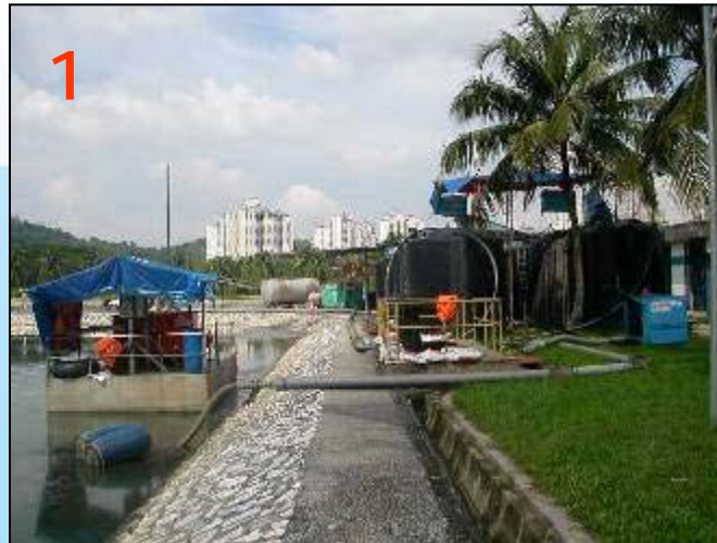
Pumping of Sludge to Treatment Facility
