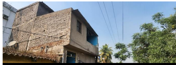
Housing with toilet (privately built) but no piped water
