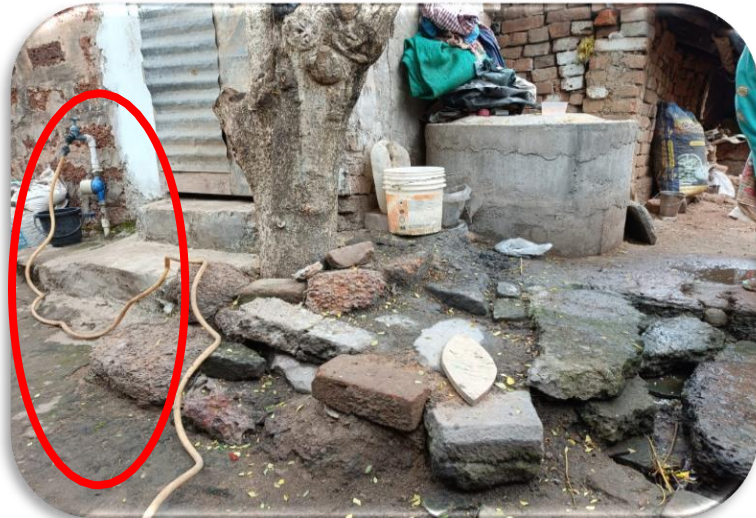
Raised water pipeline connection platform in Ward 5
