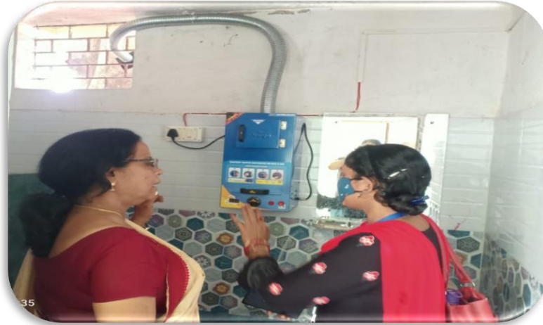
Safe sanitary pad disposal incinerator, Syed Mumtaz Ali School
