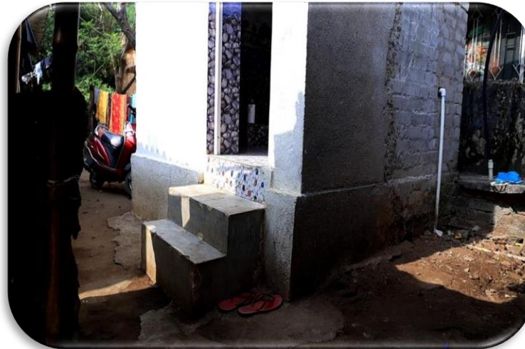
Raised toilet in Ward 43 slum
