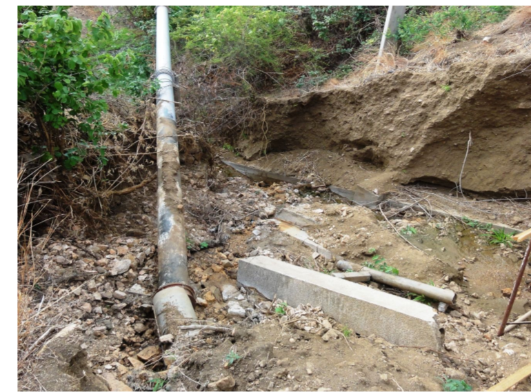
Fig . Failure of Modern System
