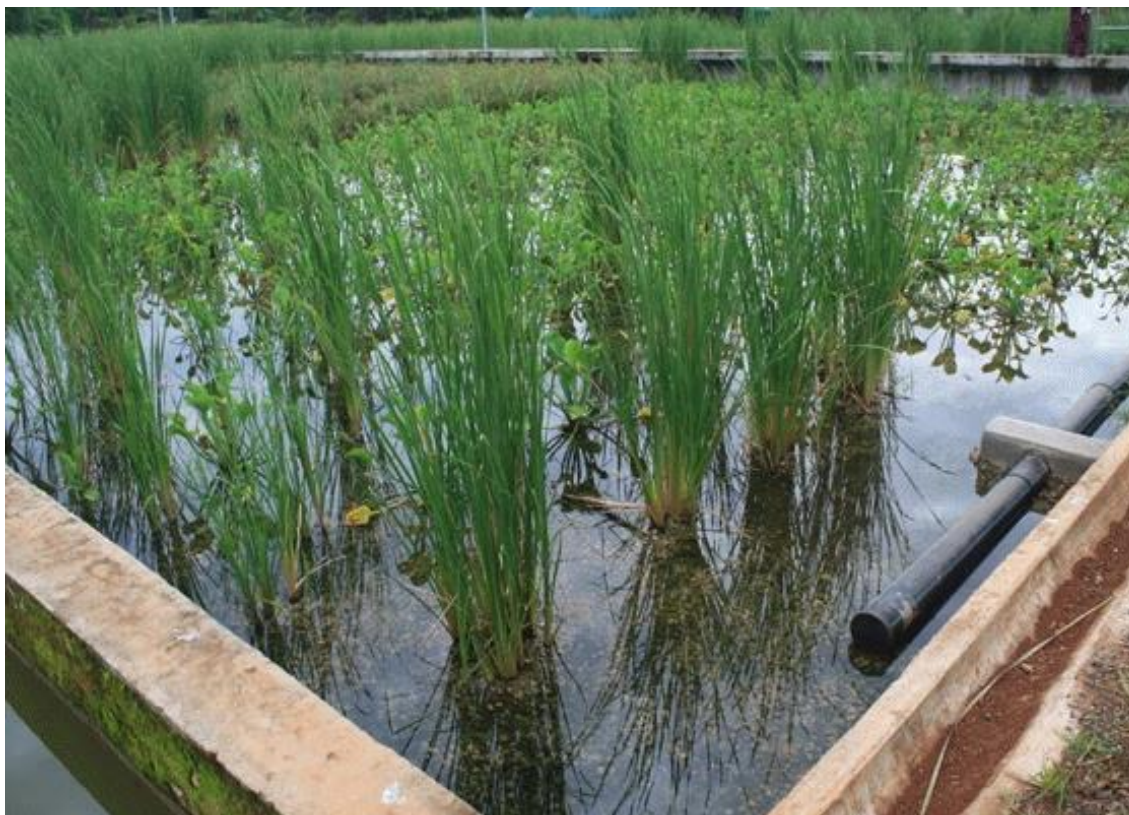
Figure 3: A Horizontal Flow Constructed Wetland (CW), with cattail planted
